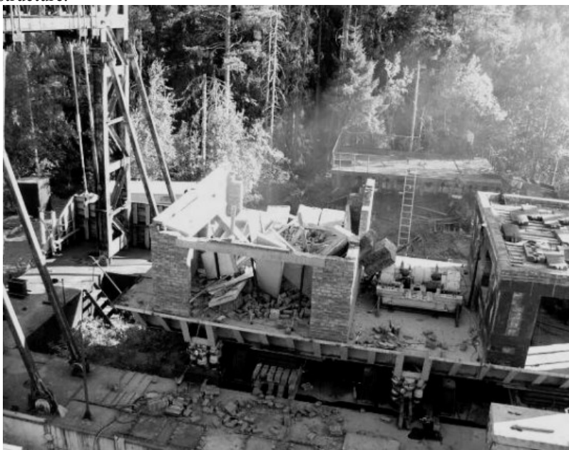
Figure 4 – Collapse of a test fragment not reinforced with composite materials. Scientific and technical statements of the St. Petersburg State Polytechnic University. 1 '2013
